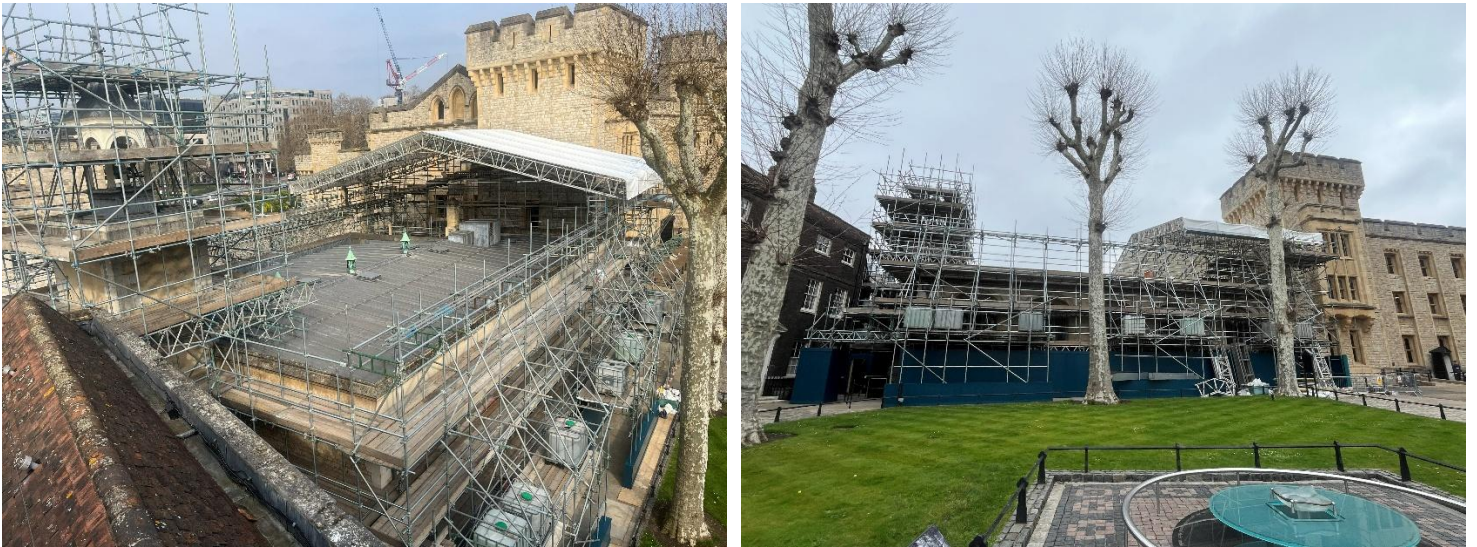
Scaffolding across the roof and on the south side of the chapel.
